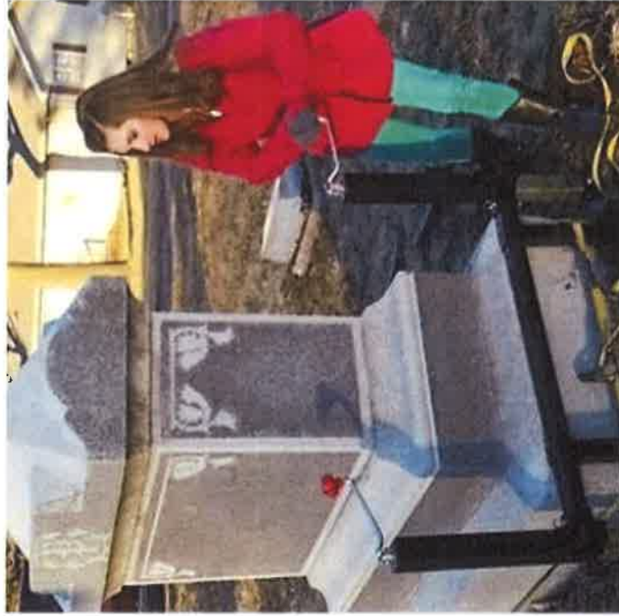
16-year-old Emily safely lifts this 7,900 lb. monument off the ground, using the lift feet for a new gravel foundation.
